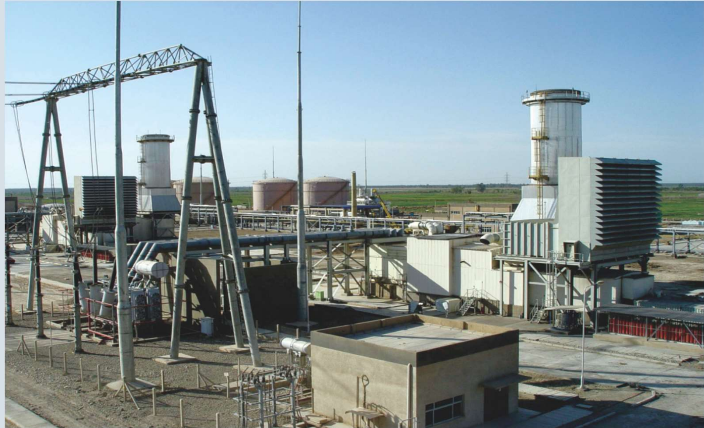
Baghdad East 4×123MW Gas Turbine Power Plant, COD in 2002
